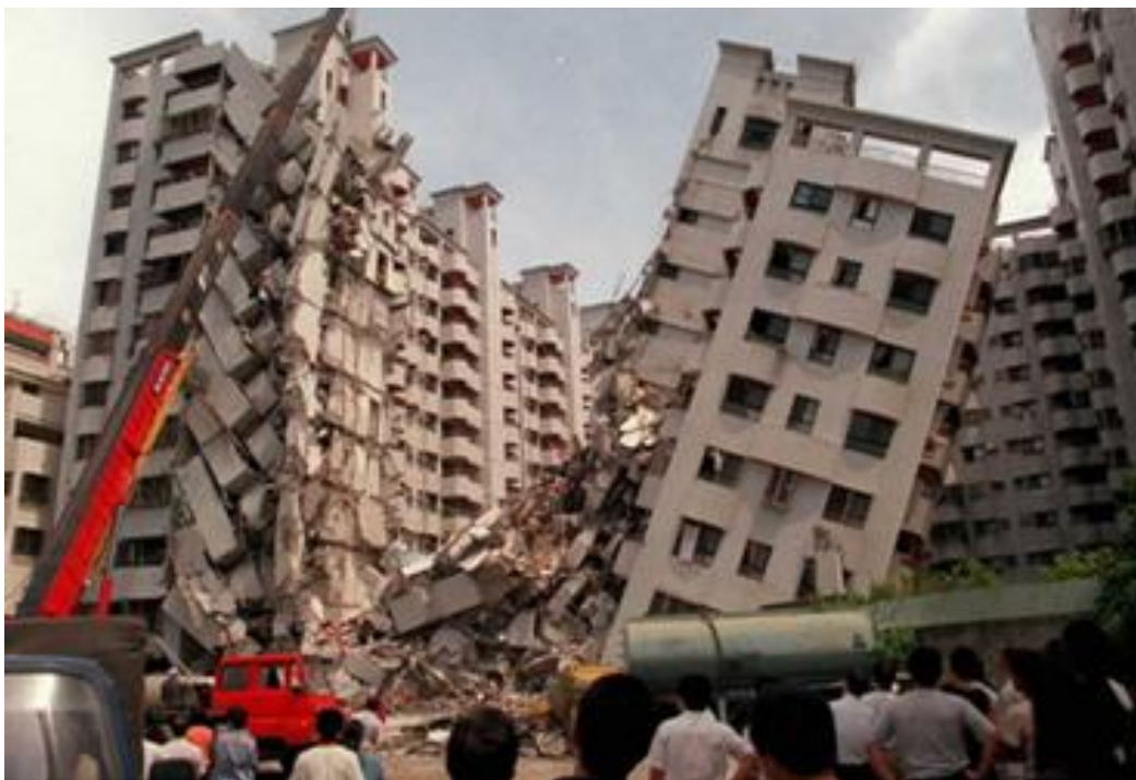
(b) Actual building damage pattern (Pixnet, 2010)
