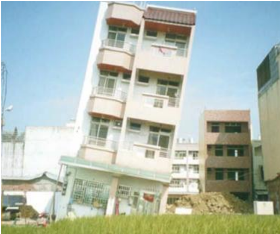
(b) The case of misidentifying the local shear failure of foundation as soil liquefaction (Moh et al., 2000)
