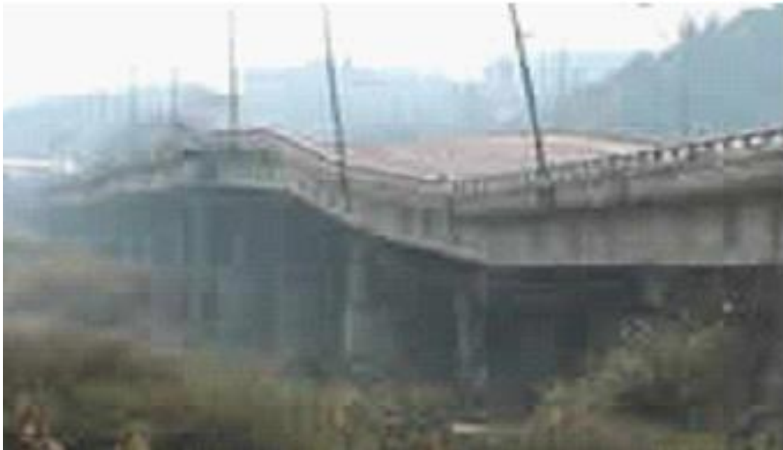
(b) Induced by the 921 Jiji tectonic earthquake (the Wu-shi Bridge)
