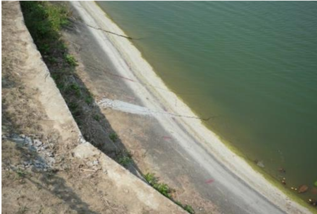
(a) After the 2010 Jiaxian Earthquake
