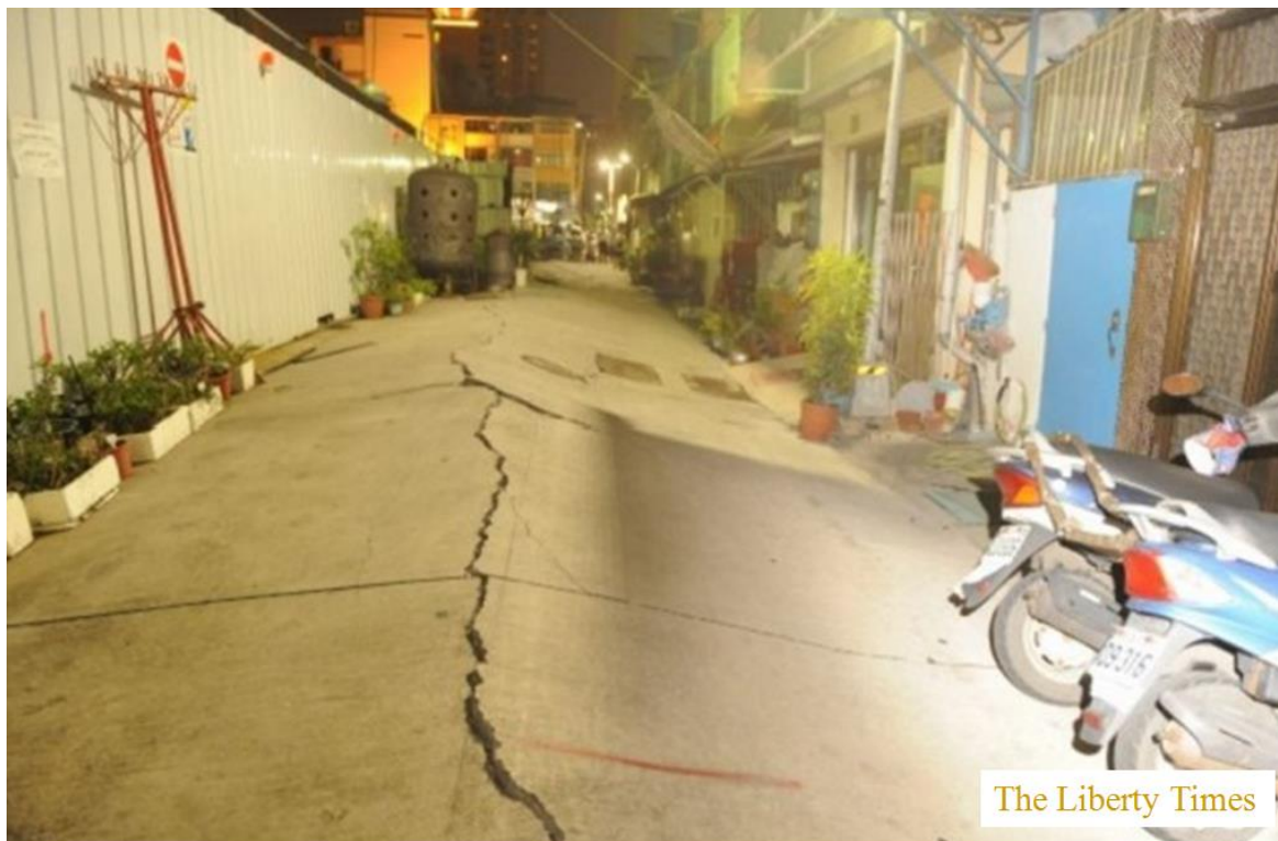
(a) Cracking on neighboring roads
