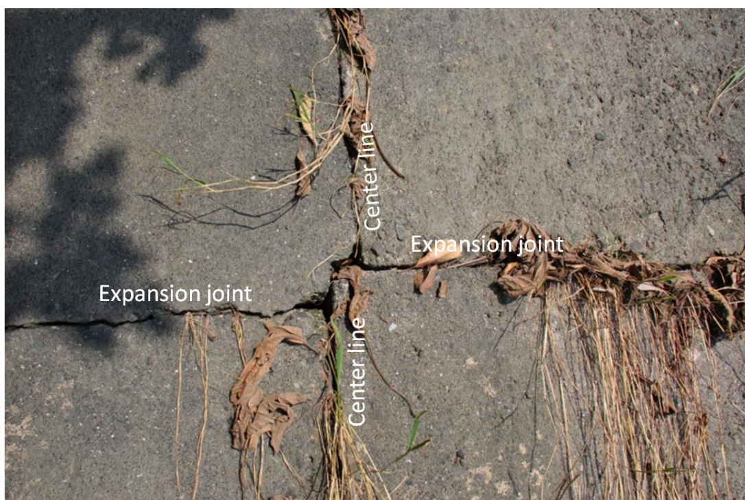
Figure 3.69. Dislocation of the center line and expansion joint of the bottom plate of Renyitan Reservoir spillway
