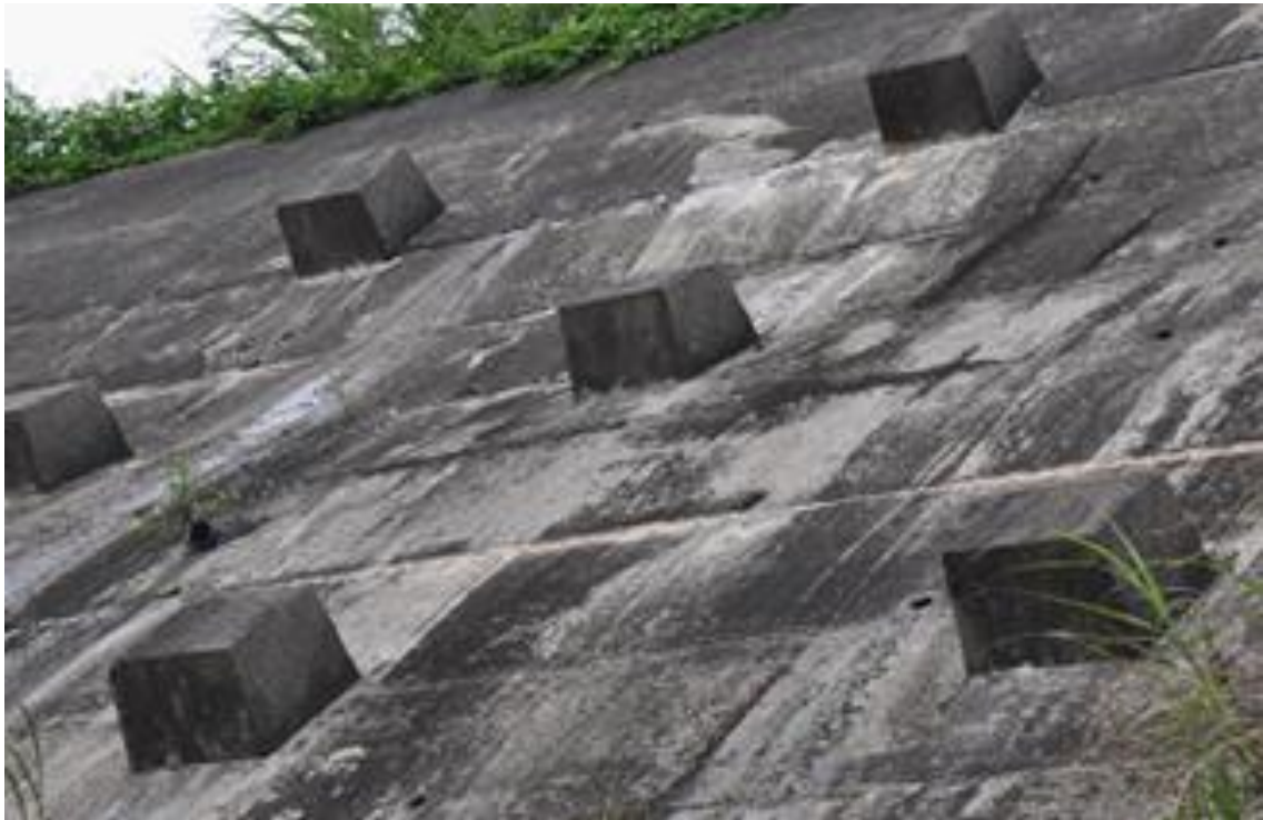
(c) Warping of the retaining wall
