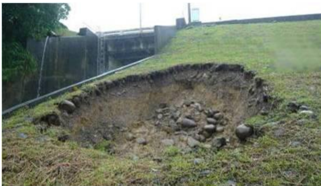
Figure 3.50. Big holes appeared on the top of the left side wall of the 3rd bottom plate
