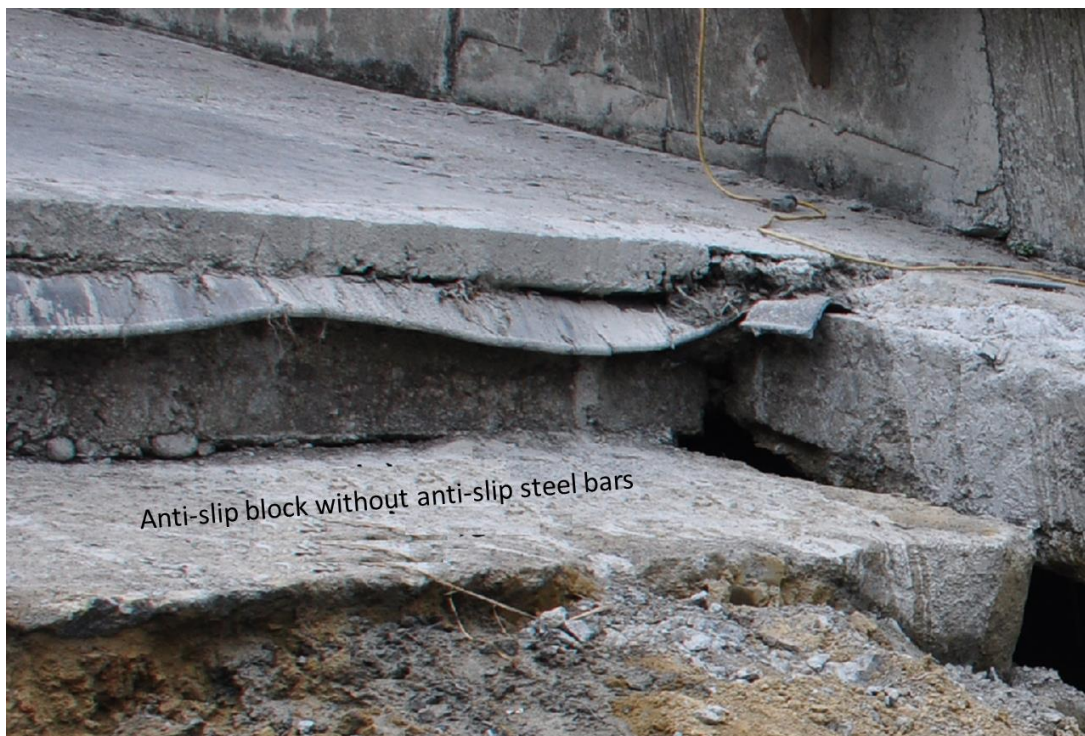
(a) Anti-slip block without anti-slip steel bars prior to the repair project
