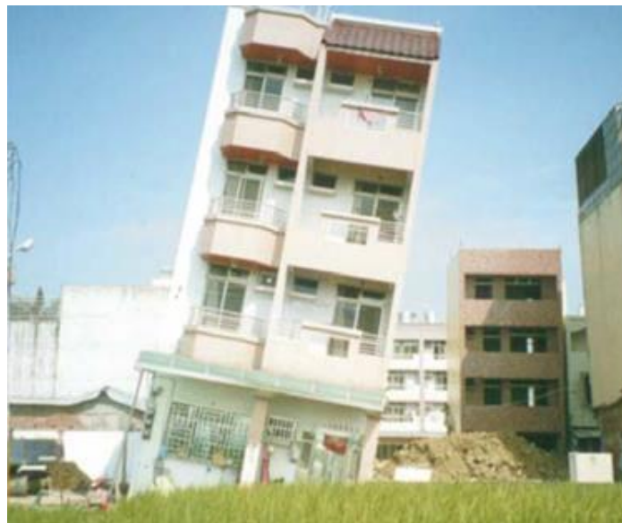
(b) The case of misidentifying the local shear failure of foundation as soil liquefaction (Moh et al., 2000)
