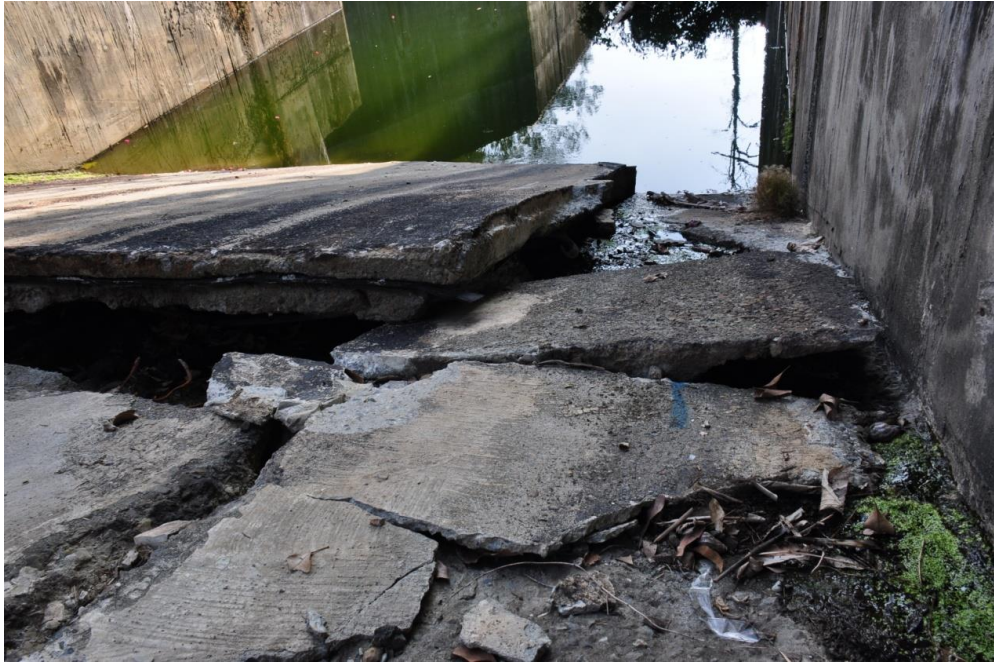
Figure 3.48. The damage to the 6th bottom plate and side wall foundation plate of the spillway
