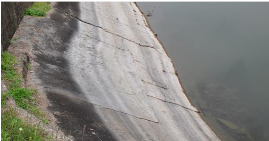
(b) After the 2016 Meinong Earthquake
