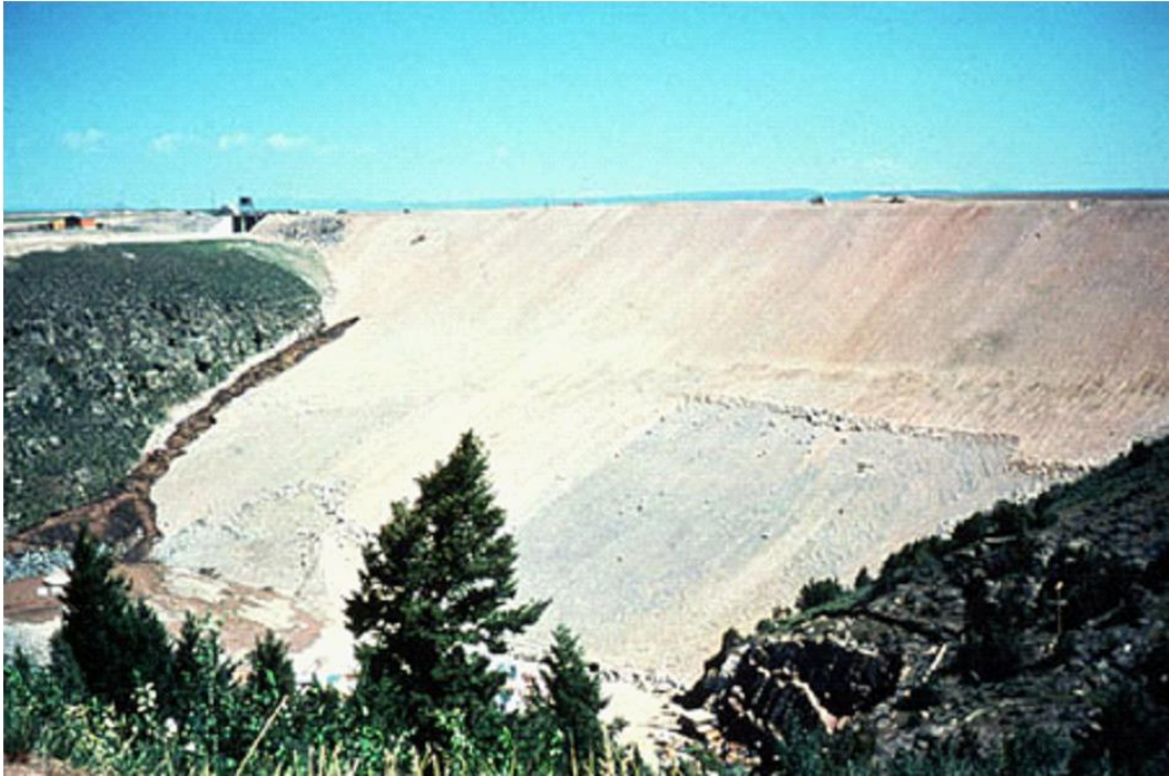
(a) Continuous leaking
