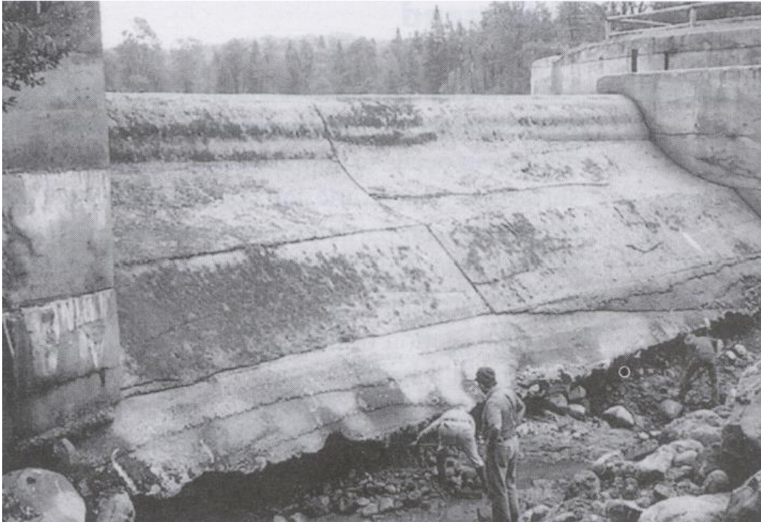
(a) The undermining phenomenon at the toe of a dam
