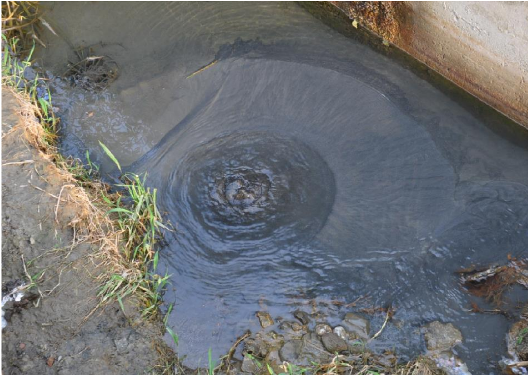
Figure 3.14 Water leakage in the downstream slope of A-kung-tien Reservoir
