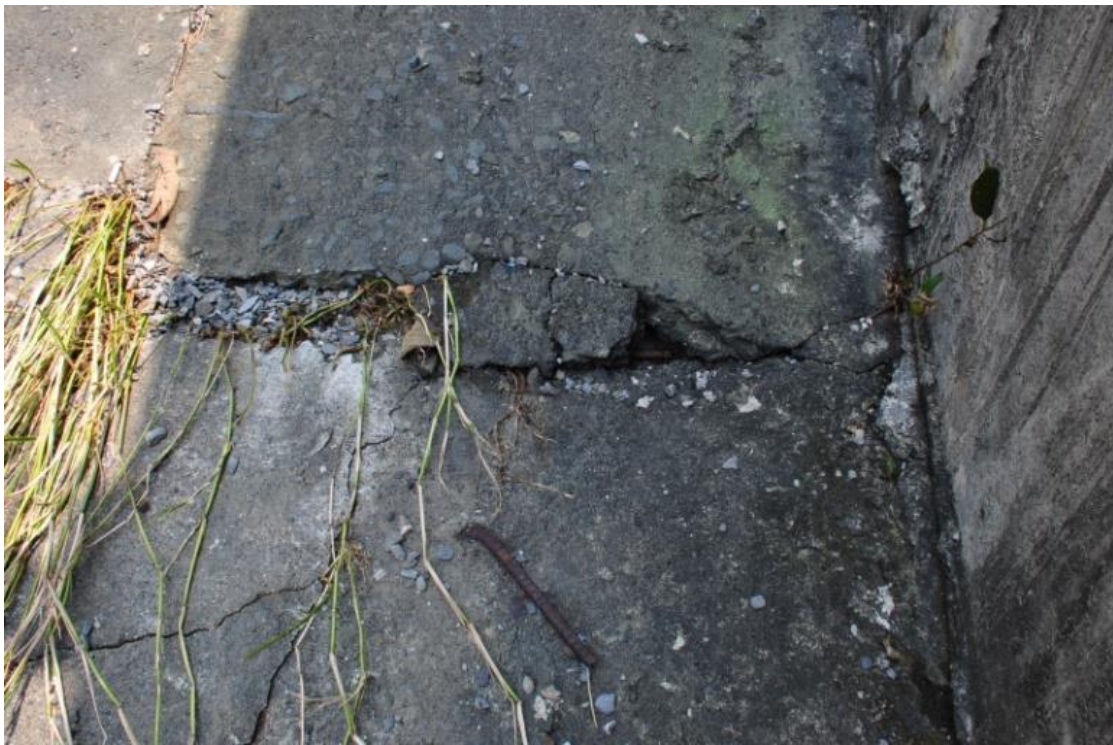
Figure 5.3 Side Wall Foundation Rupture
