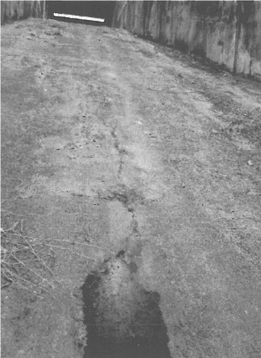
(b) Groundwater seepage after the spillway bottom plate rupture
