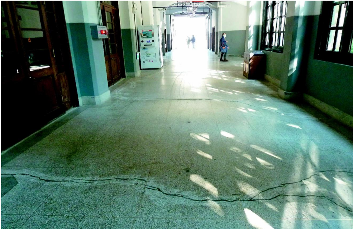
Figure 4.2. The cracking phenomena in neighboring buildings caused by construction of the Taipei Dome project in Songshan District of Taipei City (Zhou, 2017)
