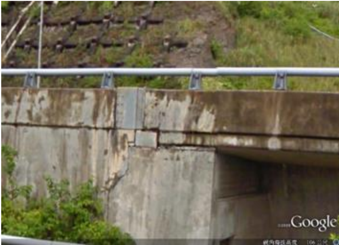
(b) Cracking of the bridge abutment
