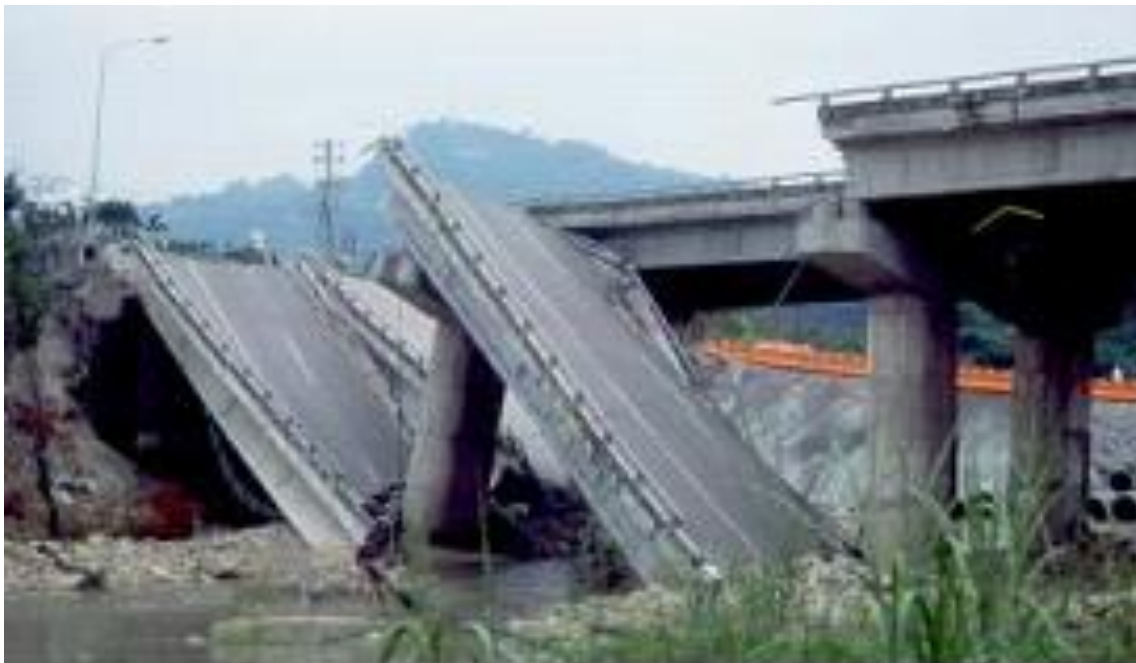
(b) Induced by the 921 Jiji earthquake (the Shih-wei Bridge, Taiwan)
