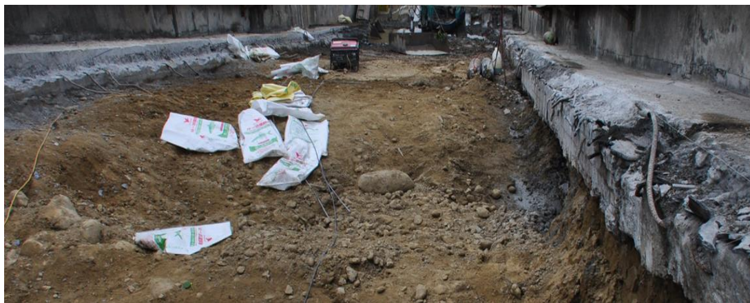
Figure 3.63. The space after the soil loss of the spillway bottom plate
