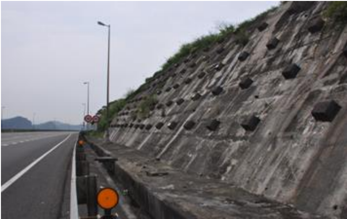
(a) Severe leaking out of the cemented substances
