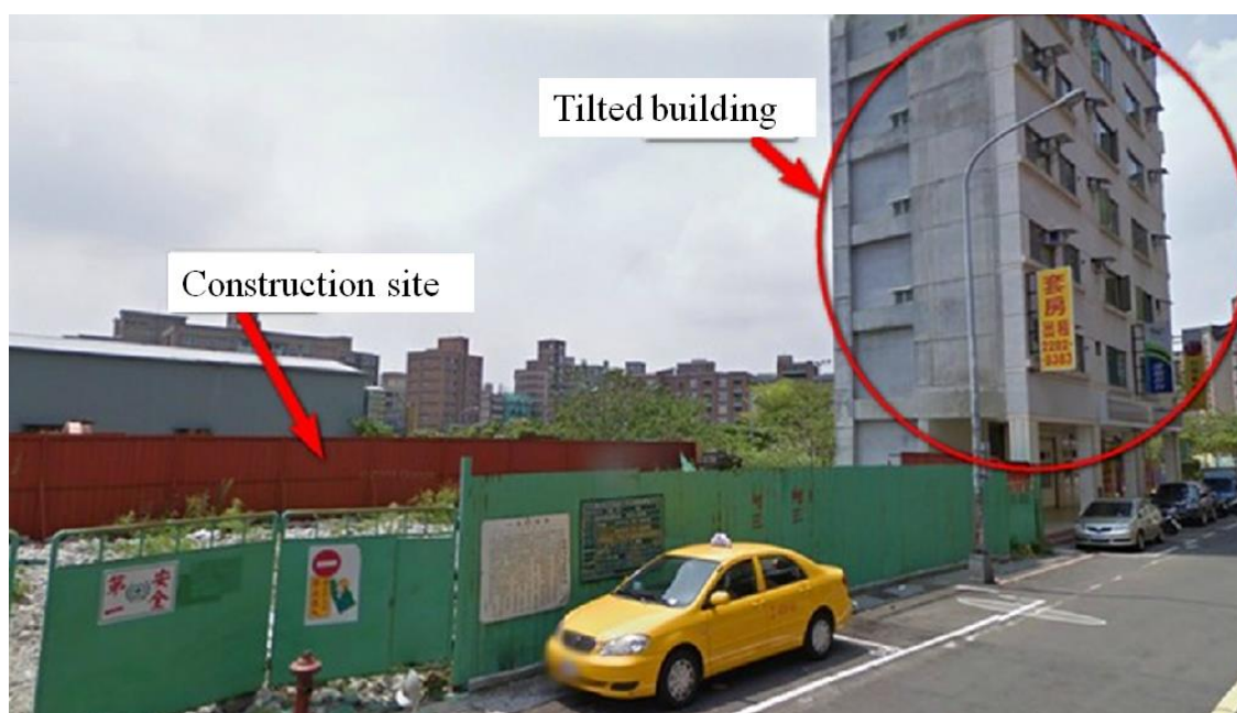
Figure 4.1. The leaning phenomena in neighboring buildings caused by construction in Luzhou District of New Taipei City (background picture is from Wang, 2012)
