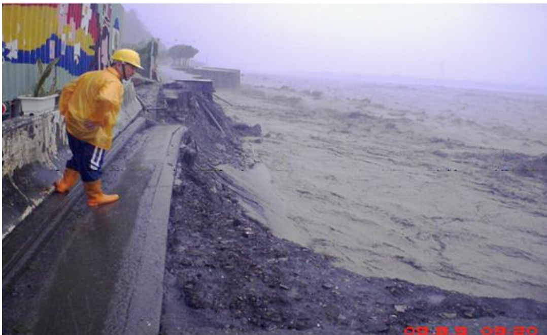
Figure 4.56. Erosion phenomenon of a shear banding river bank
