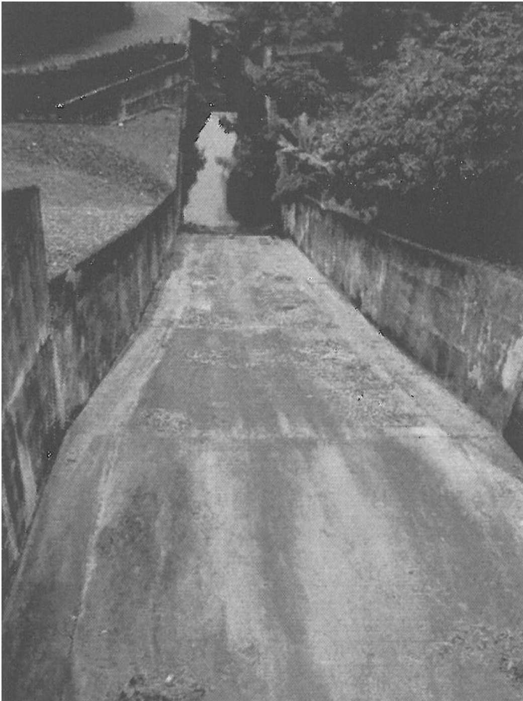
(a) The whole picture of spillway bottom plate cracks, side wall dislocation, and side wall foundation plate cracks
