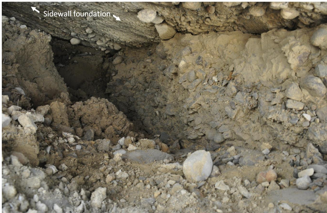
Figure 3.64. The space after the soil loss of the spillway sidewall foundation
