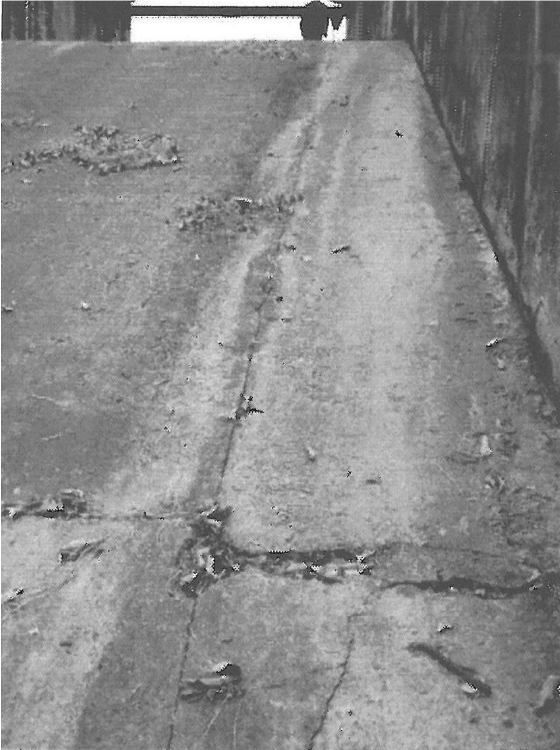
(c) Groundwater seepage after the extrusion cracks of spillway bottom plate and side wall foundation plate, as well as between the side wall foundation plates
