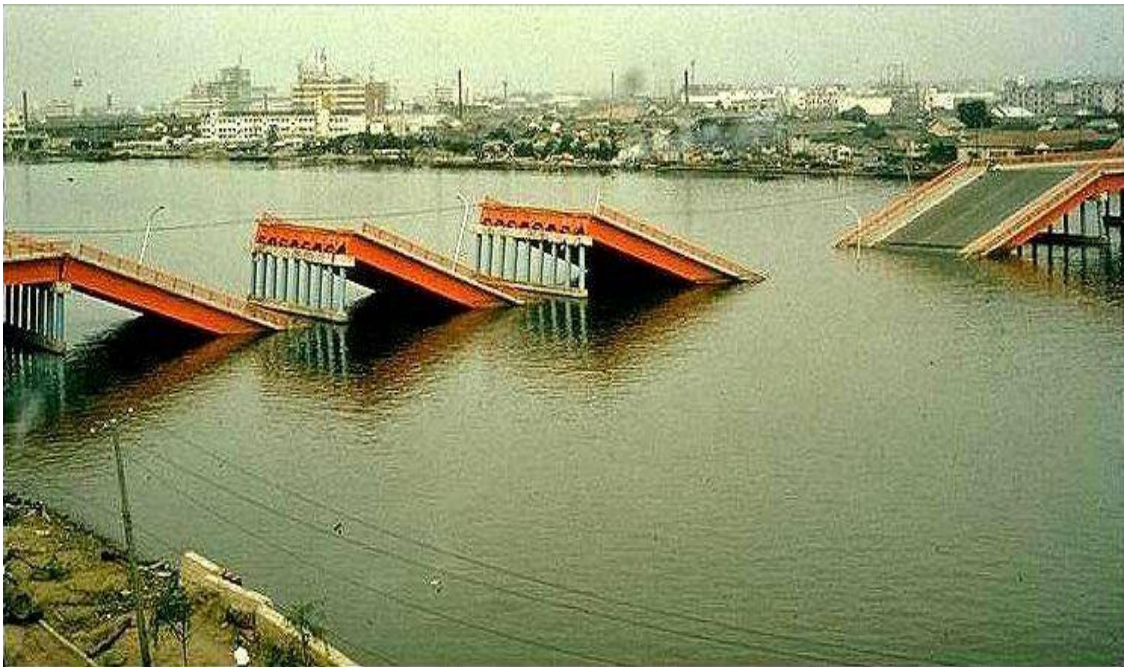
(c) Induced by the 1964 Niigata tectonic earthquake (the Showa bridge, Japan; Wikipedia, 2017 )
