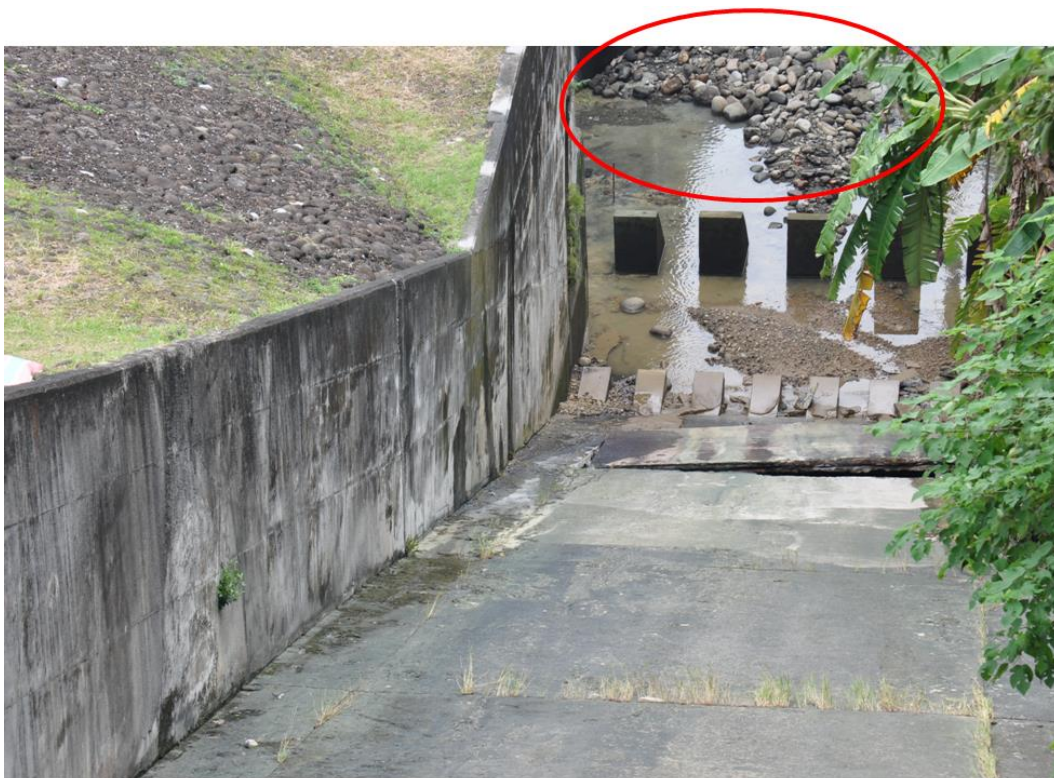
Figure 3.62 Soils of different sizes flowed out due to piping failure of Renyitan Reservoir spillway
