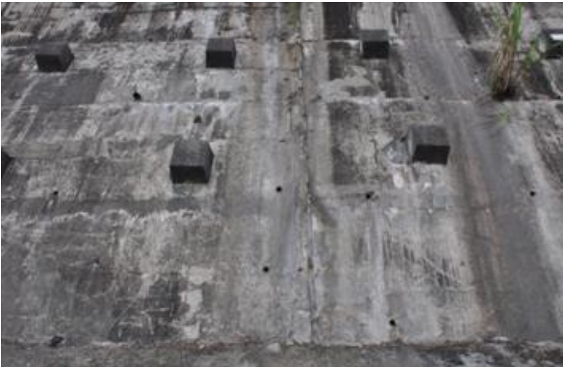
(b) Cracking of the retaining wall
