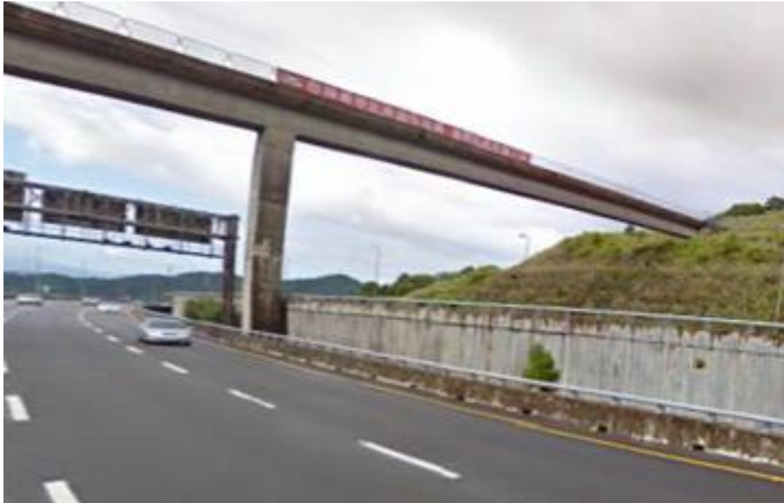
(c) Bending of the bridge
