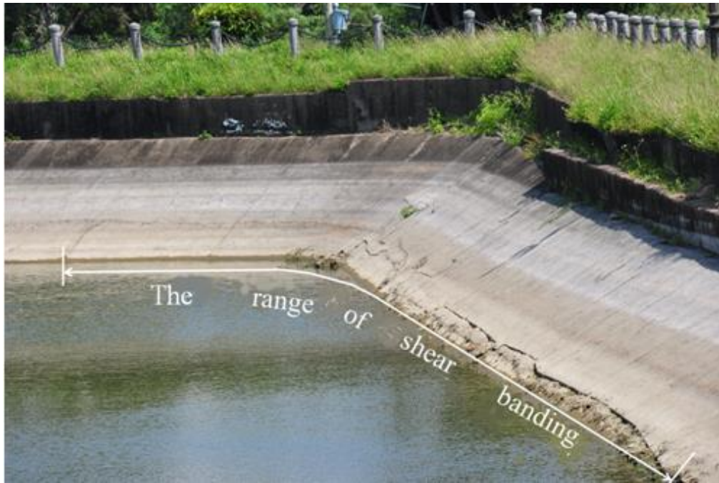
(b) The dam perimeter needs to be repaired.
