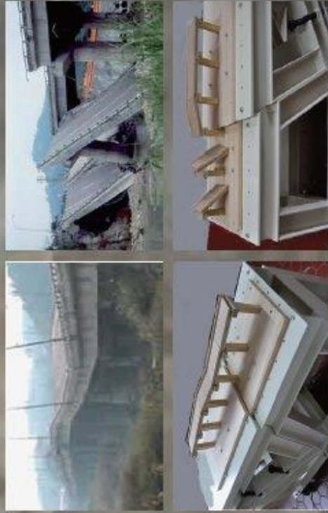
Bridges Damaged in the 921 Jiji Earthquake
