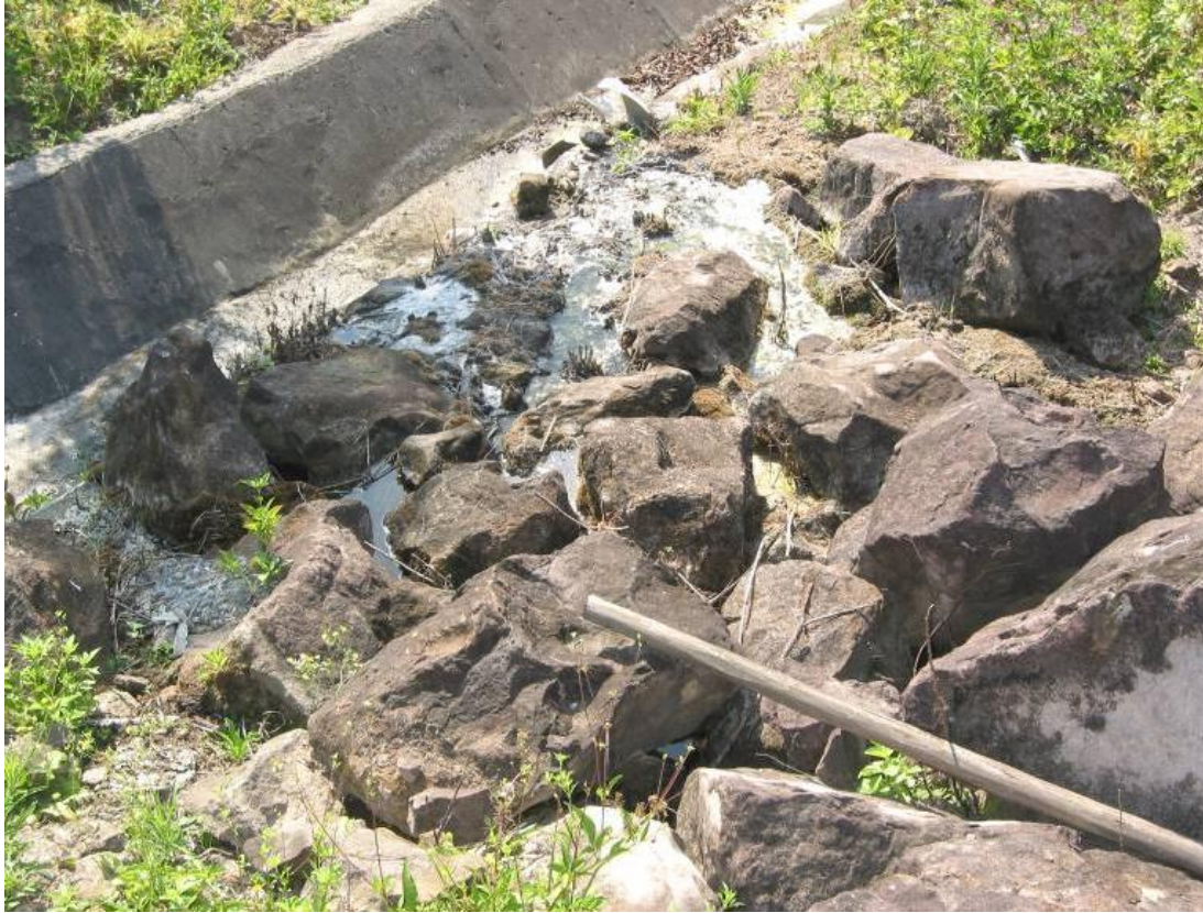
(c) Local leakage conditions II
