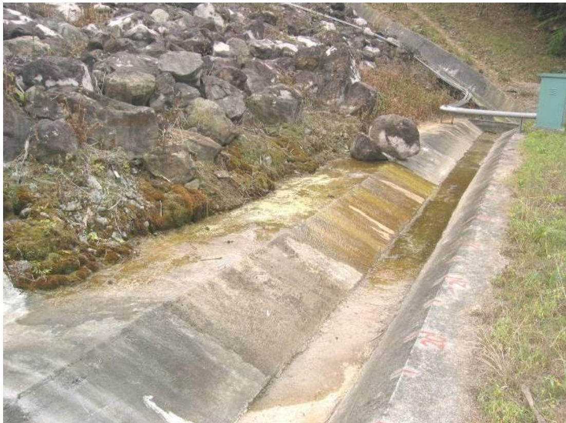
(b) Local leakage conditions I
