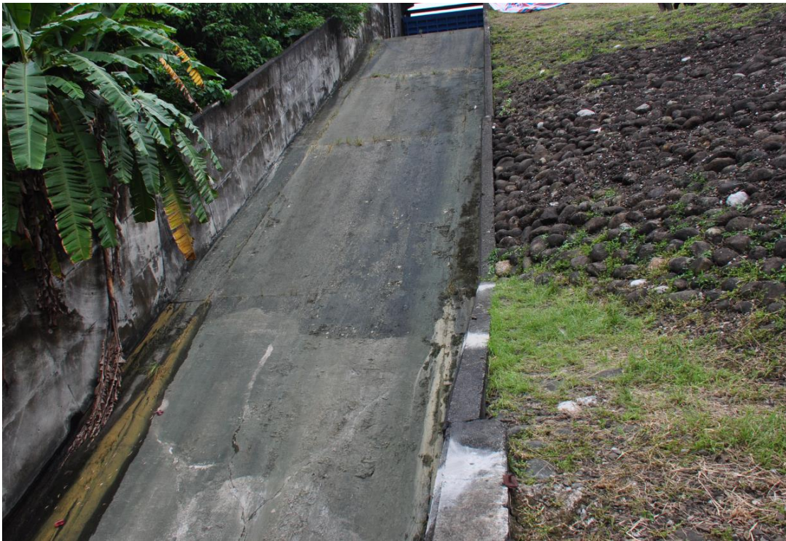
Figure 3.60 Bottom plate rupture and bending deformation of the side wall of the spillway for Renyitan Reservoir
