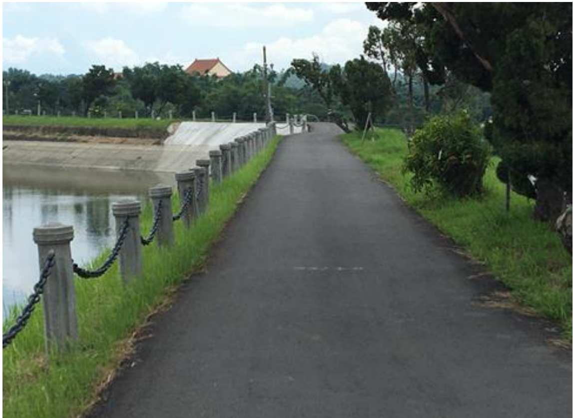
(b) AC road surface on the crest of the dam after emergency repair
