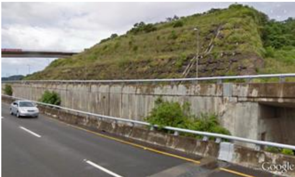
(a) Severe leaking out of the cemented substances
