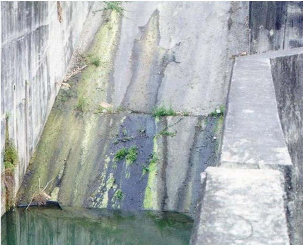
Figure 3.61 Dislocation of the side wall of Renyitan Reservoir spillway
