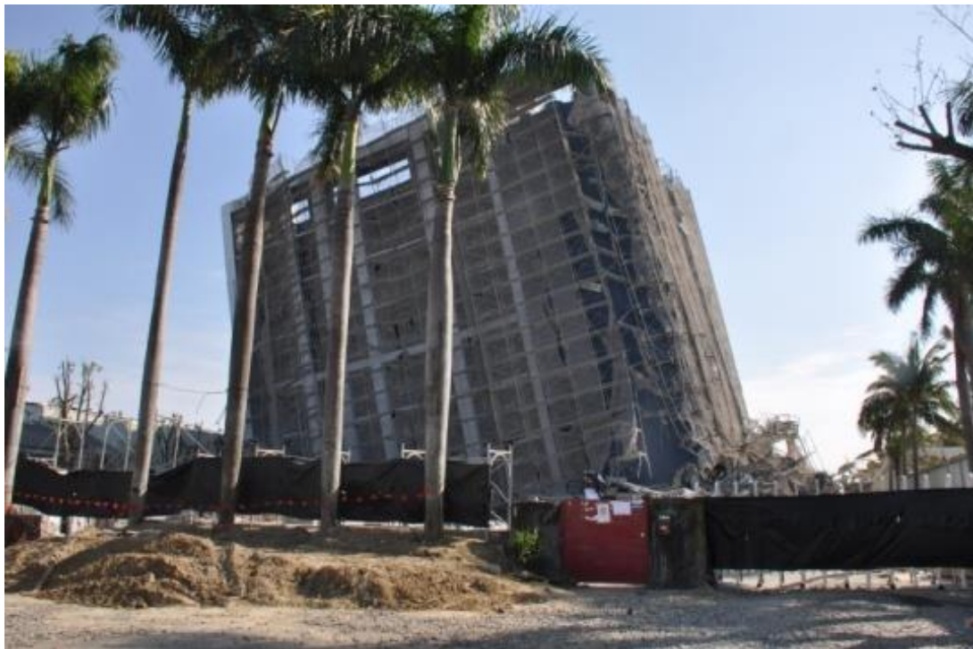
(b) After the tilting damage
